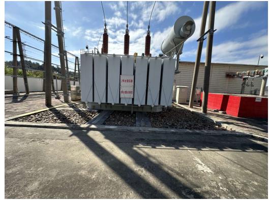
现有 2 号主变 (50MVA)
